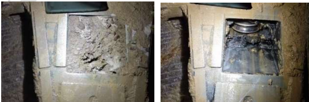
Figure 18. Clogging of disc window due to the injection of bentonite powder (left), Cleaned up disc window (right)
