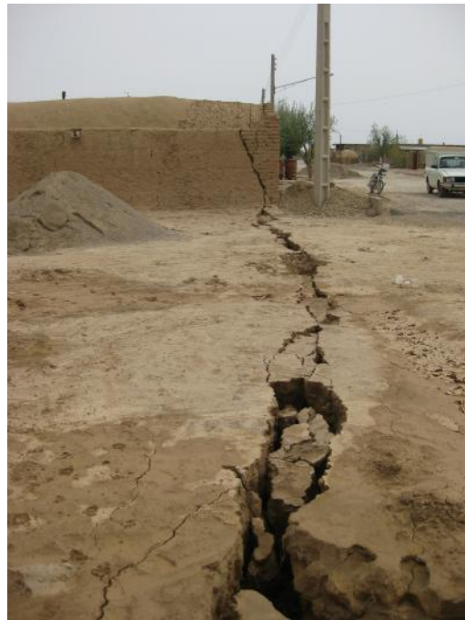
Figure 13. Photo of a long wide crack formed due to land subsidence south of the Damghan plain
